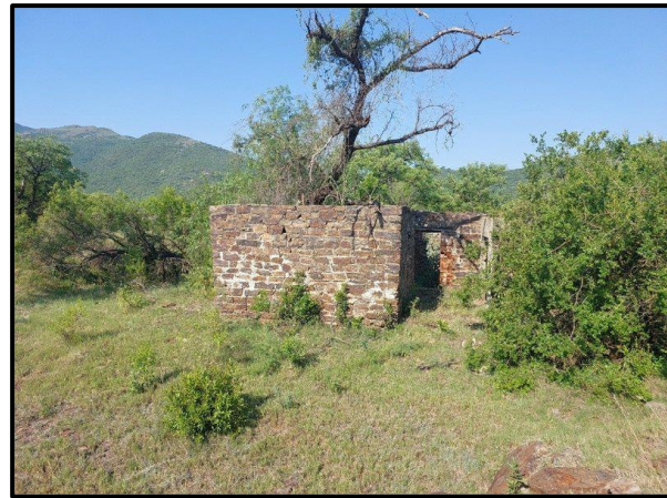
Figure 7.9. Ruin 3 - The structure is mostly still intact with the doors, windows and roof having been removed.
