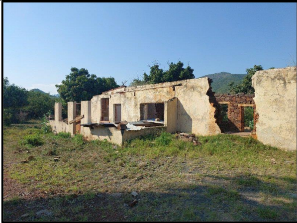
Figure 7.10. Historical Farmstead - General view of the large historical farmstead situated at the top of the small hill at the centre of the application area
